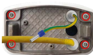
Fig. 17: Installed and ready for Connector Box LSA
