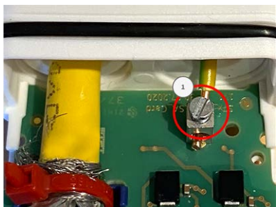
Fig. 15: Ground wire connected to terminal
