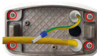
Fig. 12: Installed and ready for Connector Box LSA
