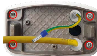
Fig. 17: Installed and ready for Connector Box LSA
